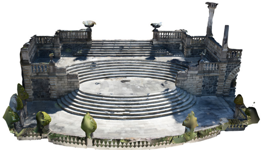
FIGURE 4. Staircase of the Jardín de las Pérgolas, MNH. 3D model elaborated by digital photogrammetry (Survey and elaboration of the model: Áyax Horacio Segura Galván, January 14, 2023; courtesy: Museo Nacional de Historia, CNMH).
