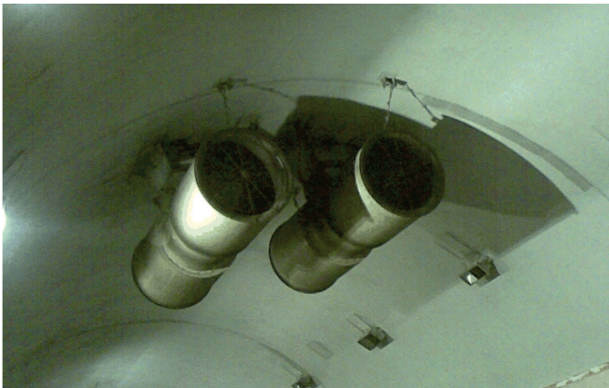
Fig. 8. Installed SDS112T-4P-22 jet fans in tunnel.
